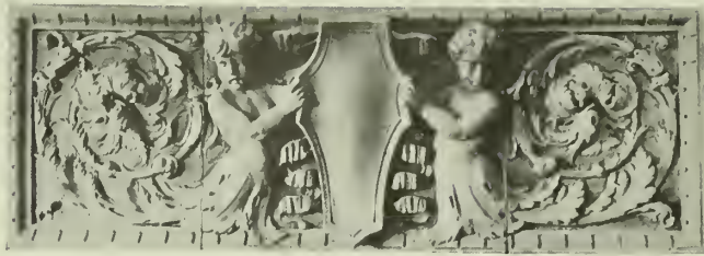
DETAIL BY GOLDWIN STARRETT & VAN VLECK, ARCHITECTS. New York Architectural Terra Cotta Company, Makers.
